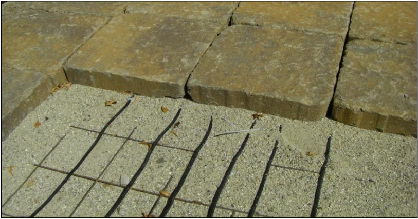
Example of insufficient sand on top of cables.
