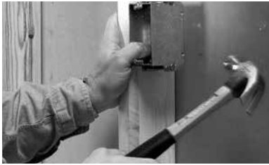
Figure N2. ECB installation
