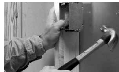
Figure 1a. ECB installation
